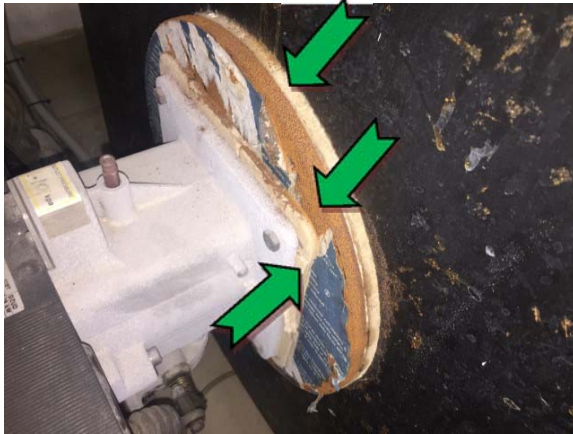
Photo 1. Pump plant room, west elevation, to boiler – non asbestos-containing packer, woven material and gasket.
