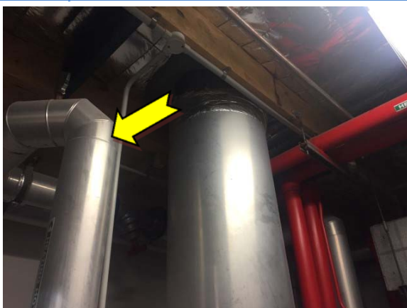
Photo 5. Interior, pump plant room, pipework – suspected internal SMF insulation.
