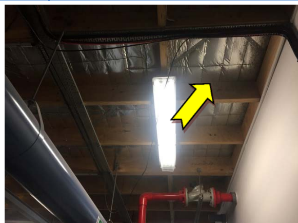
Photo 6. Interior, throughout, ceiling – suspected SMF sarking insulation.
