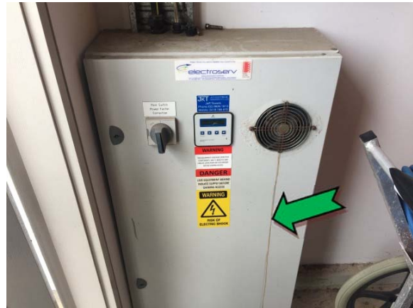
Photo 4. Interior, main switchboard room, switch power factor corrector – suspected non asbestos-containing bituminous backing board.
